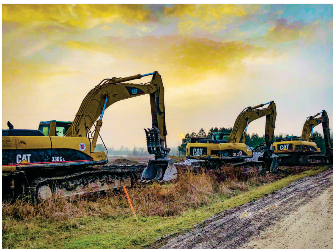
Heavy construction equipment sits idle along the edges of Highway 411 due to a recent rainy day in Cherokee County. Work began in earnest late last year on the long-planned four-laning of the final five-mile stretch of Highway 411 between Leesburg and Gadsden. The project is expected to take up to five years to complete. PHOTO BY LEANN HILL
