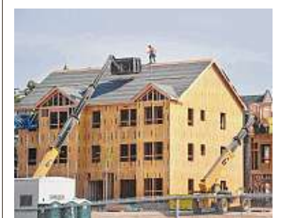
Construction of housing in Bridgeport is seen in 2020. Brian A. Pounds/Hearst CT Media
