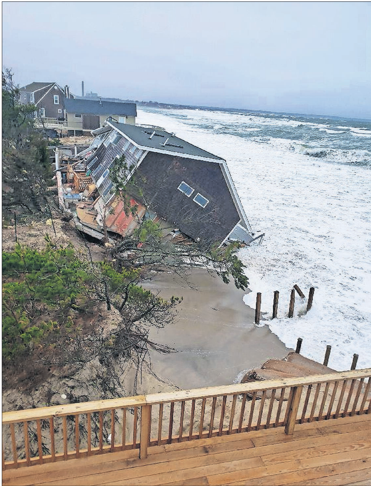
A home on Salt Marsh Road collapsed into the ocean late Tuesday afternoon. The home, which sustained heavy damage in Monday's storm, sits in an area that has been battered by beach erosion over the years. [PHOTO COURTESY OF MIKE POTTEY]
