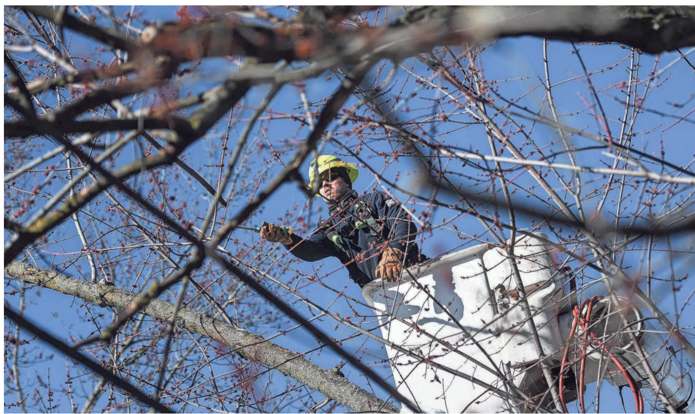
Lansing Board of Water & Light certified arborist Cory Caswell cuts branches above utility lines on March 15. PHOTOS BY MATTHEW DAE SMITH/LSJ.COM
