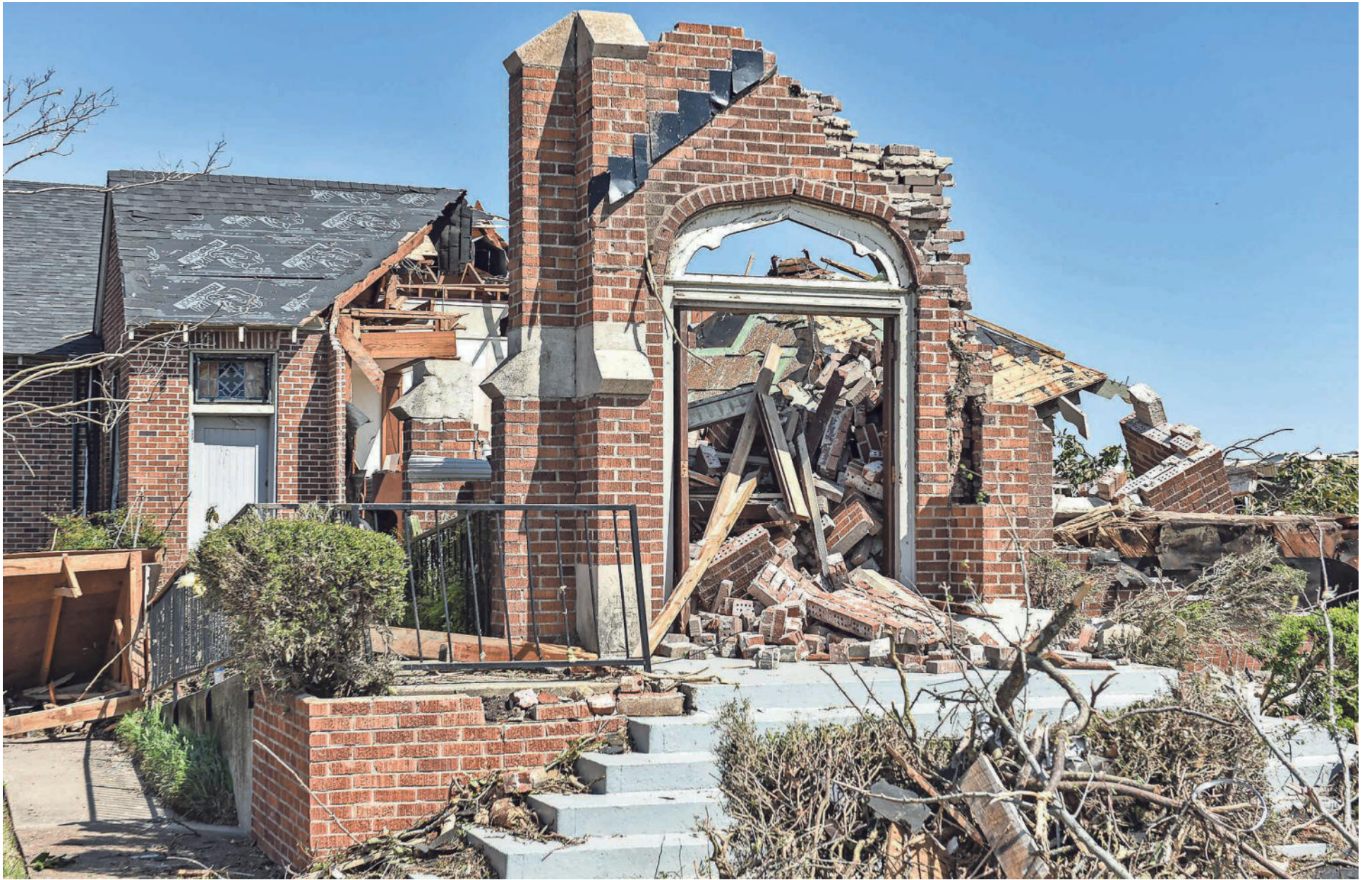
What remains of the Chapel of the Cross Episcopal Church is seen in Rolling Fork on Sunday. PHOTOS BY HANNAH MATTIX/CLARION LEDGER
