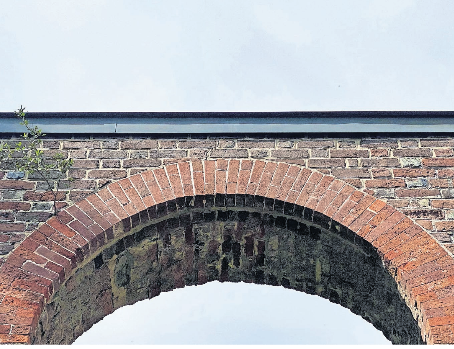
A crack (center) in the top of the arch of St. Philip’s Church at Brunswick Town/Fort Anderson State Historic Site in Winnabow is believed to be damage done by a tornado during Hurricane Isaias in August. [HUNTER INGRAM/STARNEWS]
